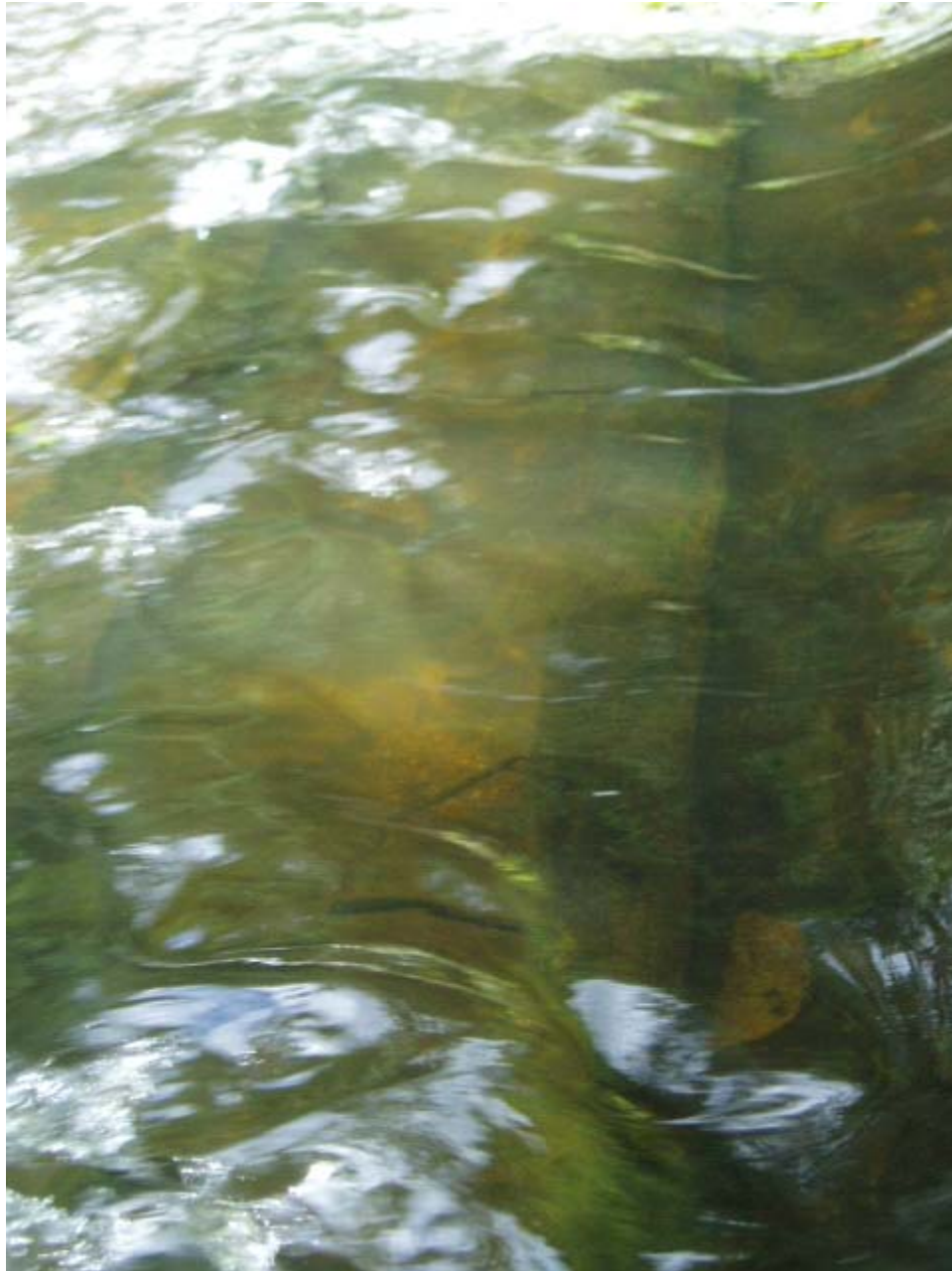
Photo 15. Close up view of Eagle Mill Dam remnants. Note cribwork alignment perpendicular to channel alignment and large metal spikes.
